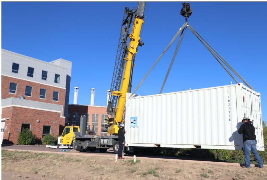
Dr. Bryan Willson (left) and Kirk Evans (right) guide one of the two hydrogen station fuel containers into a temporary location at the CSU Energy Institute Powerhouse Campus. Payment keypad visible on the side of the container
